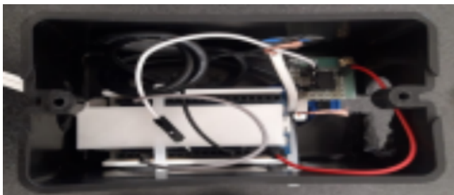
Figure 2. SM inserted in an electrical box.
