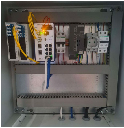
Figure 2. OT network electrical panels, housing the industrial switches and optical fiber ring terminations that support the plant's communication infrastructure.
