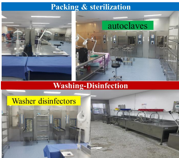
Figure 6. Equipment and installation in disinfection and sterilization zones in CSSD-UH of Oujda city.
