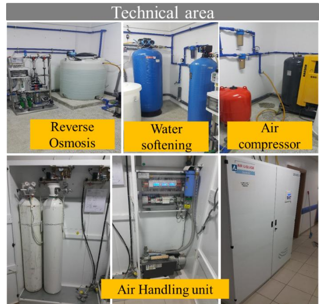
Figure 7. Equipment and installation in technical zone in CSSD-UH of Oujda city.
