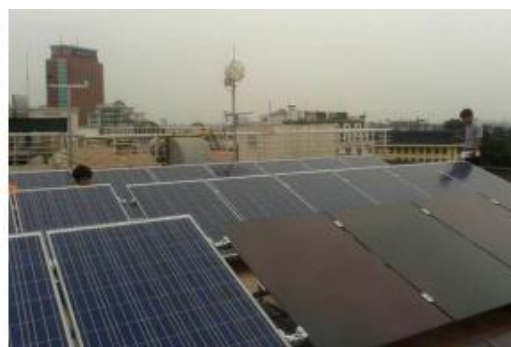
Figure 13. GDE building solar PV system [25]
