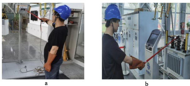
Figure 2. Testing the 10kV high-voltage constant point and aligning the high-voltage conductive rod of the transformer for phase by phase verification
